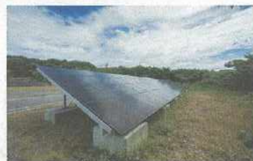
Solar panels near Gakkogura generate electricity used at the brewery, helping make its sake brewing process sustainable.
